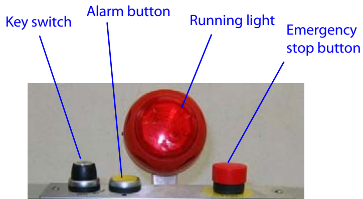
PLATFORM CONTROL PANEL
